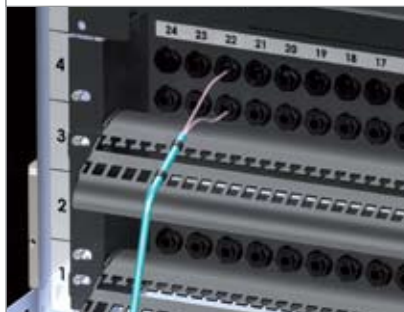
2. Close up of manifold cable entry.
